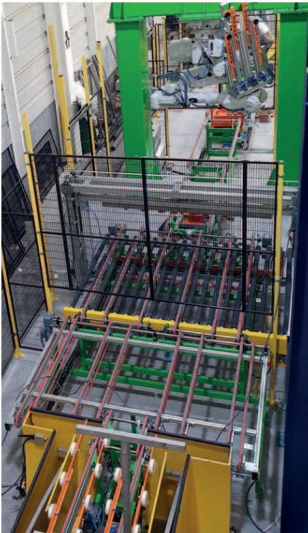
FURNACE AUTOMATIC UNLOADING
