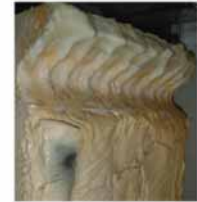
Accelerated refractory wear at metal line due to corrosive nature of foam
