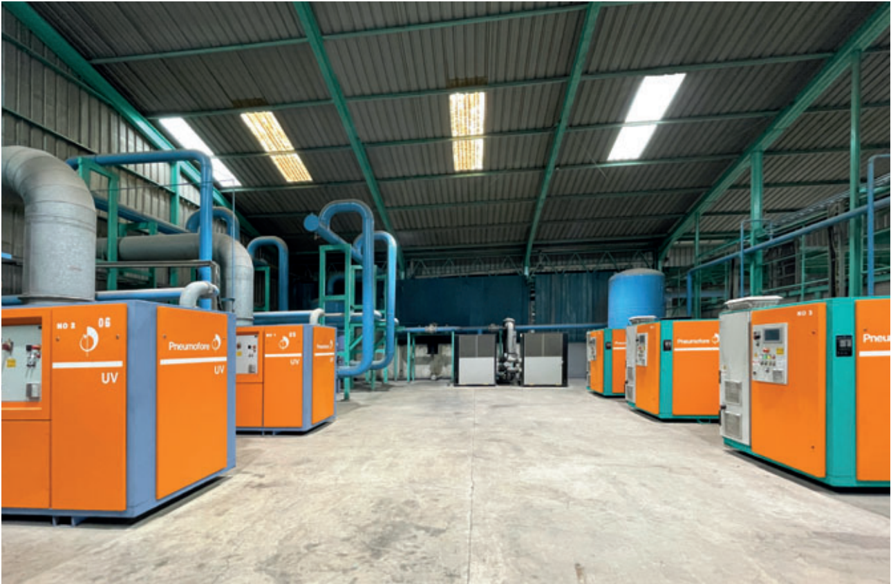
Mulia Glass, Indonesia: 3 x A180 Air Compressors, Air-cooled, Hot climate version, 160 kW each. 2 x UV50 Vacuum Pumps, Air-cooled, Hot Climate version. This customer has six more Pneumofore units installed since 2015.
